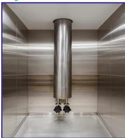
Loop System Piping (Pendants)
